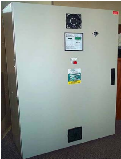
Metal Case containing Automatic Capacitor Banks
